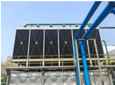
Cooling Water System
