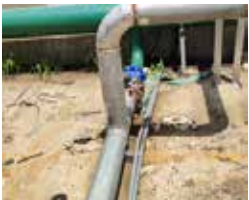
Rainwater Collection System
